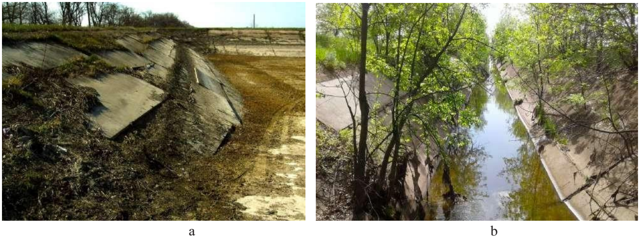
Fig. 6. Ruined areas of anti-seeping coverage at the current stage of technical exploitation of the structures: a – retention pond; b – main canal
