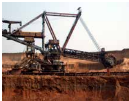
Figure 2. Selective excavation of top soil and subsoil at the open pit quarry
