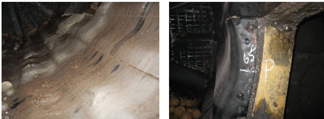
Figure 4 – Wear of linings and measurement of plate height during inspection
