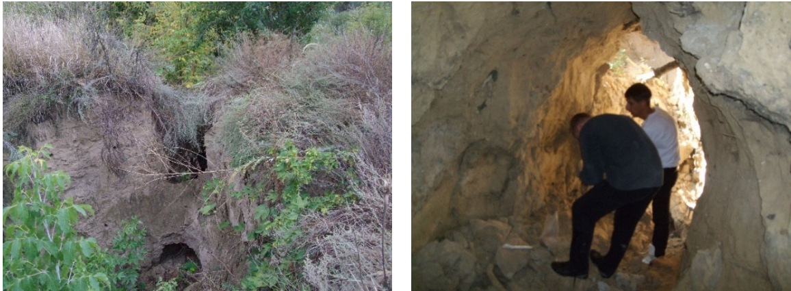
Figure 3. Manifestation of suffusion processes in the dam of the Sukhachivske tailing pond. Own photos.
